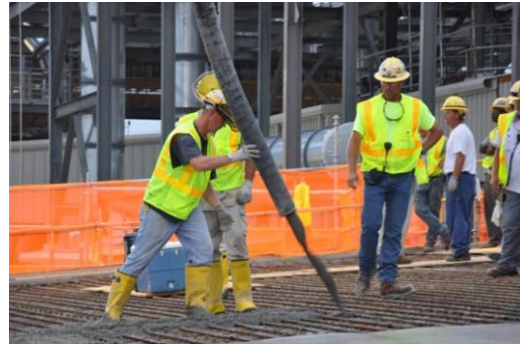
Figure 31: Delivery hose danger zone
