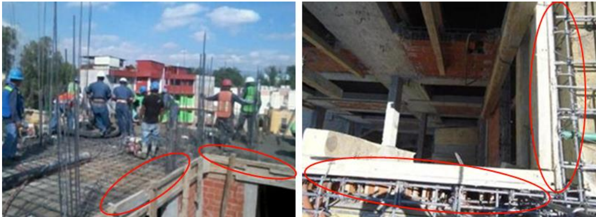
Figure K6: Site pictures showing lack of edge protection, working at height PPE and underfoot obstacles presenting a tripping hazard.
